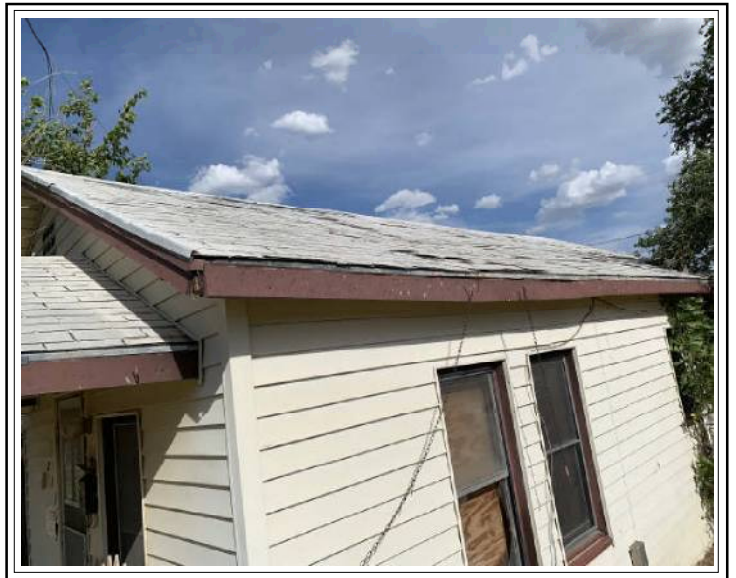
Roof damage and broken window
