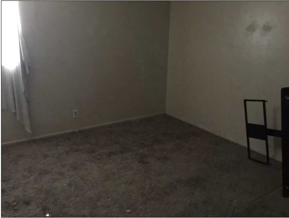
Typical interior view within one of the vacant units (to be renovated)
