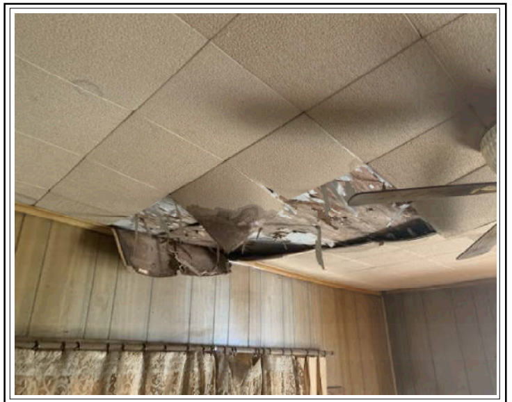
Interior Roof leak
