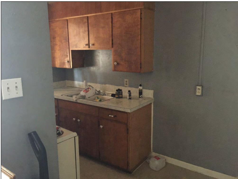
Typical interior view within one of the vacant units (to be renovated)
